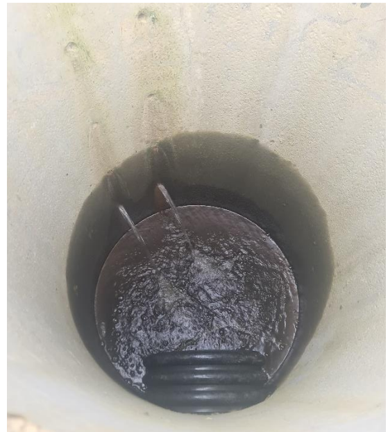
Figure 4: Paired inlet holes every 200 mm are visible with exit pipe at the bottom of the riser pipe
